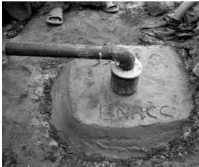
Plate 5.2 - Water harvesting borehole at Tosha
